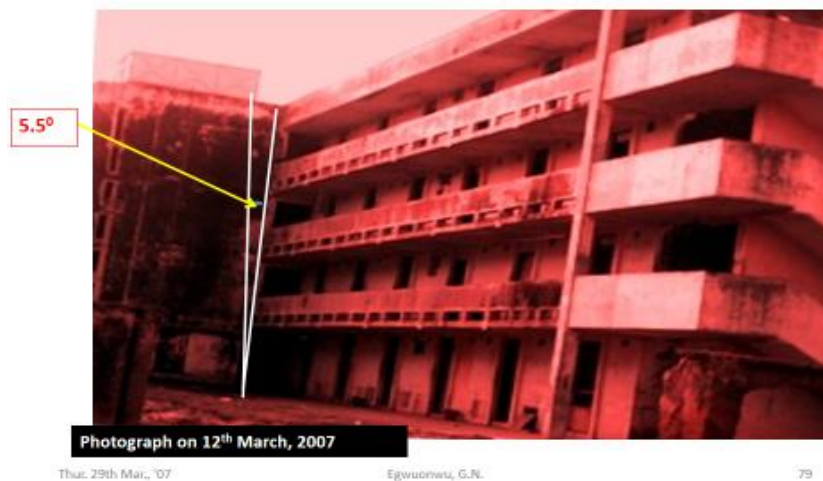
Figure 3: Seismicity leading to Earth Tremor and resulting in the tilting of the super building in 2006 at ABU, Zaria, Nigeria (Egwuonwu et. al. , 2009). This tilting would have been more severe and widespread if it were earthquake
