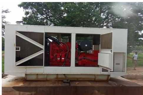
Plate 4: 500 kVA Diesel Powered Mikano Generator (Relatively New)
