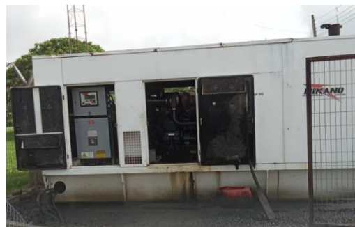
Plate 5: 500 kVA Diesel Powered Mikano Generator (Relatively Old)
