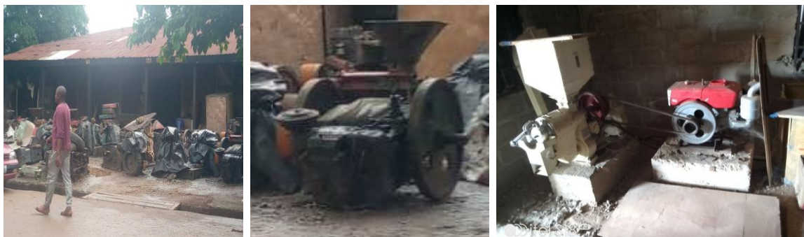
Figure 2: Diesel generators used in the cluster; images taken at the site
