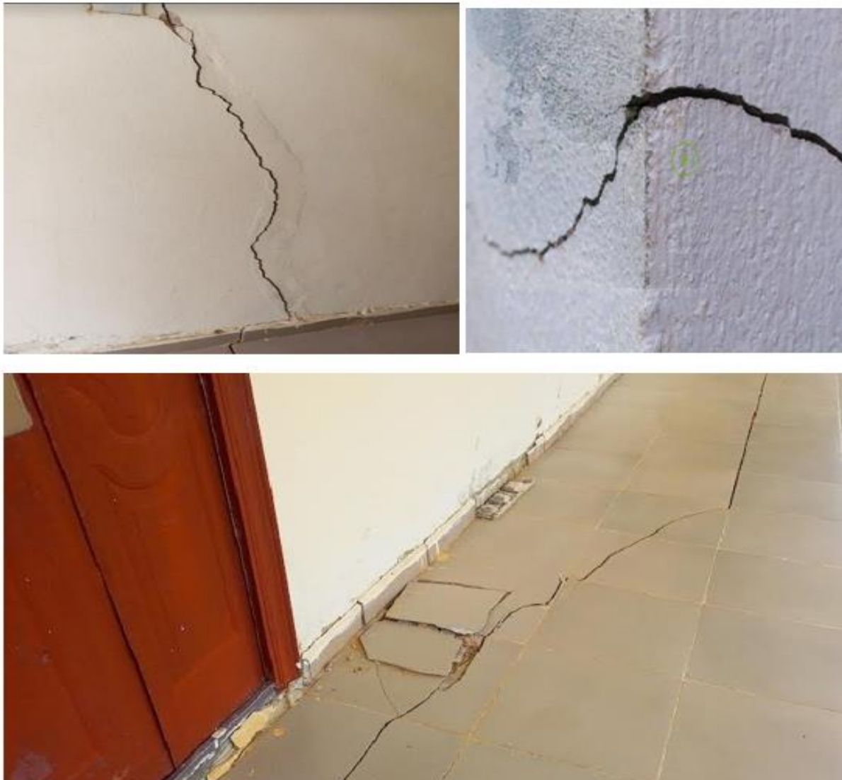
Figure 1: Common building distress leading to building failure in the study area
